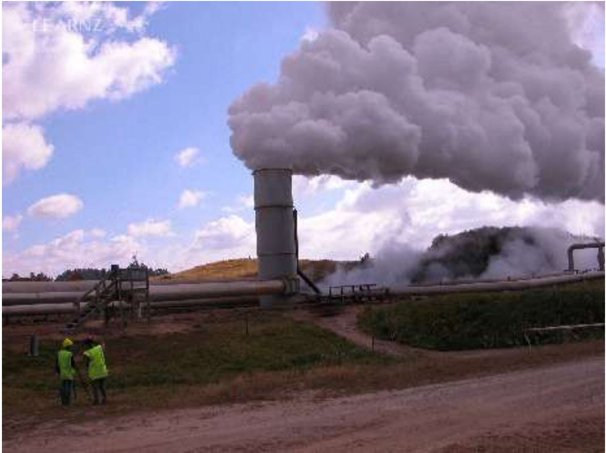
A silencer on the Wairakei field. Pressurised water enters from the left and leaves at atmospheric pressure on the right
