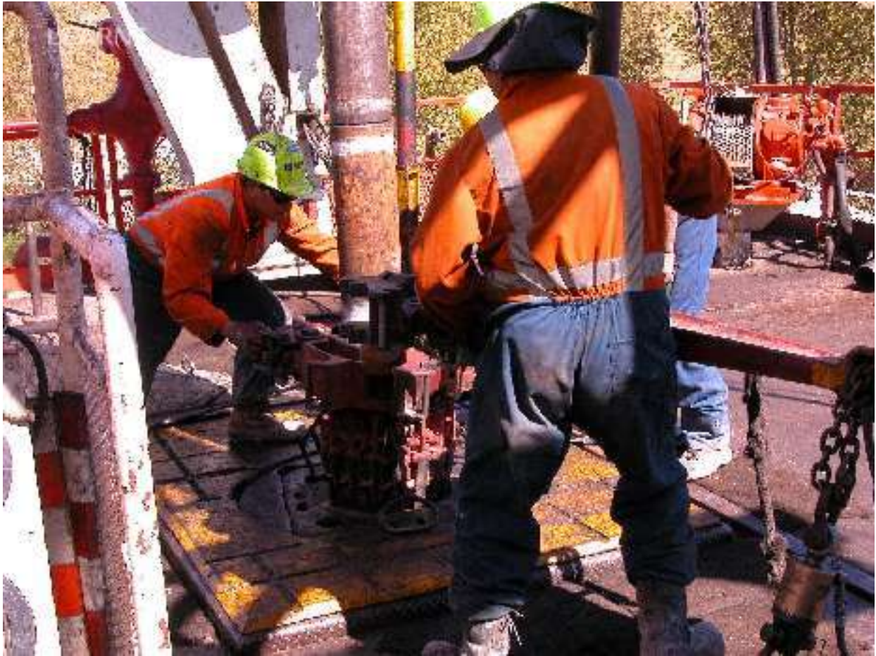
Ensuring sections of the drill string are tightly screwed together on the drill platform was a difficult, important and carefully completed task.
