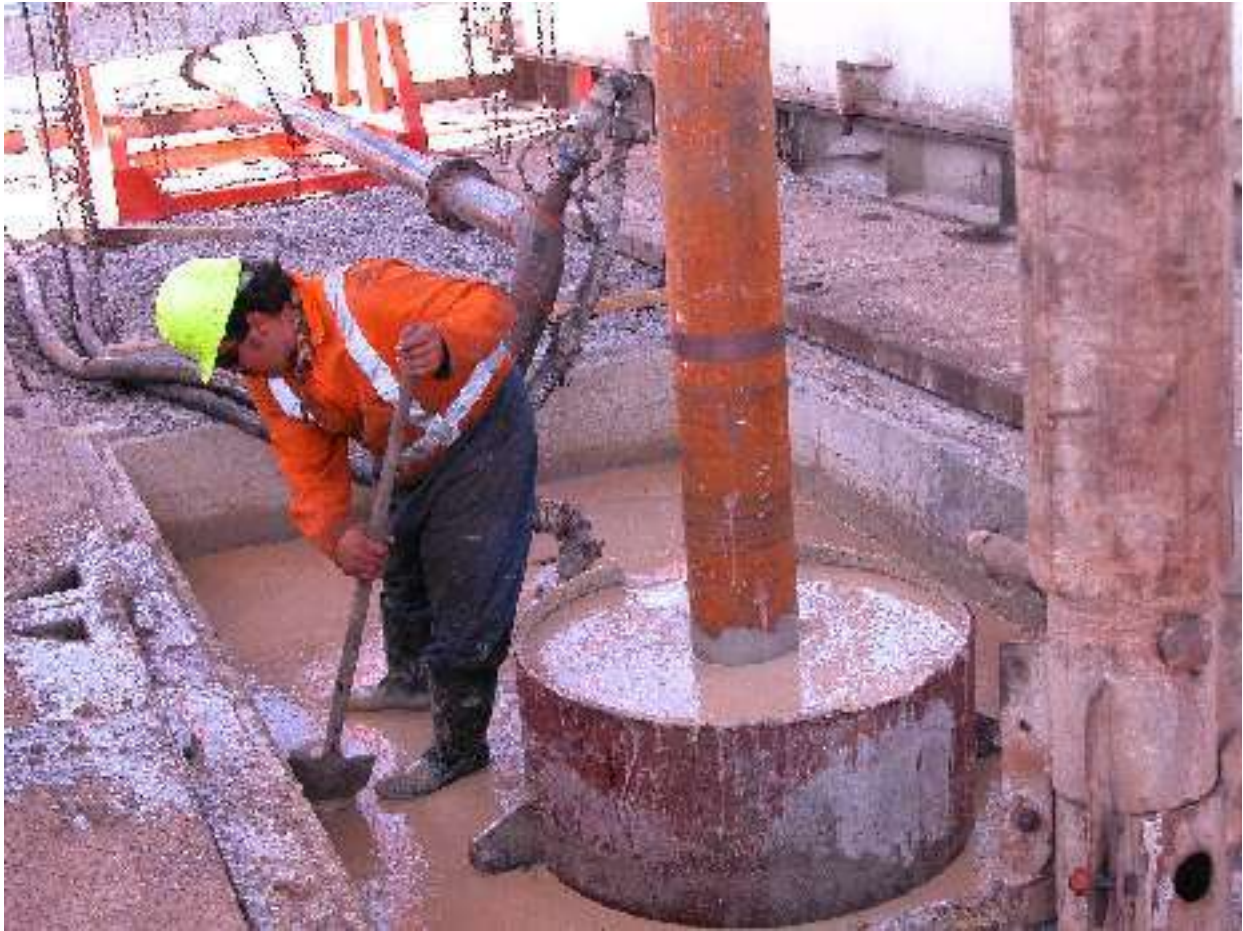
The Wairakei 248 rig has just bored 6m of its 3000m journey. Notice the drilling mud pouring back up into the well head cellar.
