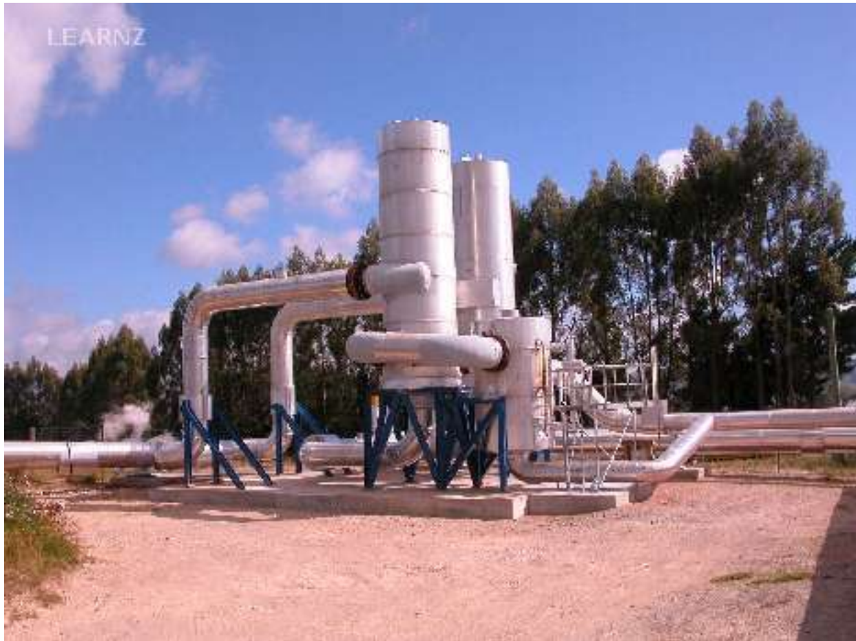
Flash plant 12 which serves several well. The steam and water mix enters on the left but leaves on the right separated from each other.
