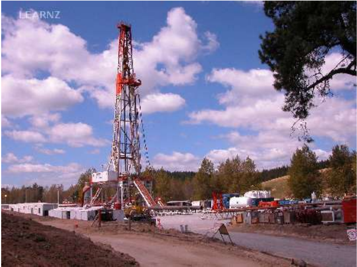
The drill site for Wairakei 248 is really a small mobile town. The rig alone weighs 500 tonnes
