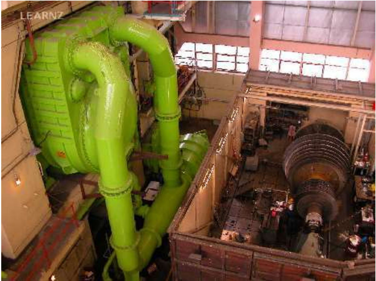
The condenser of turbine 11 is painted green to show it carries fresh water. The turbine's rotor can be seen on the right sitting in a lathe
