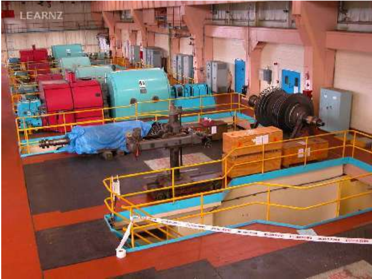
G1 and G4 are the two Intermediate Pressure turbines and generators. Note the spare generator rotor under the blue cover and spare turbine rotor to its right.
