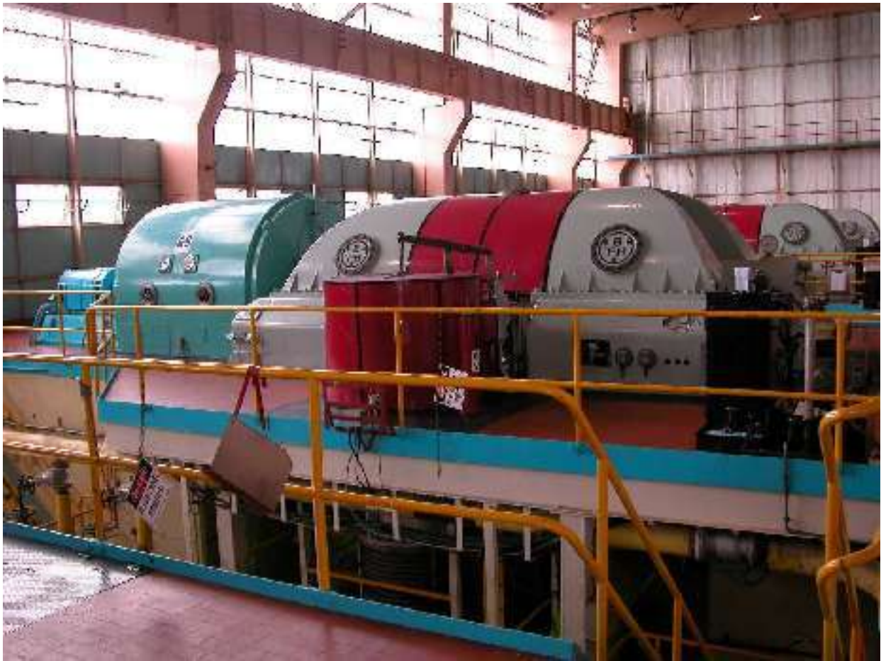
The row of Low Pressure turbines that sit high up in Station A. Their generators and exciters are to the right
