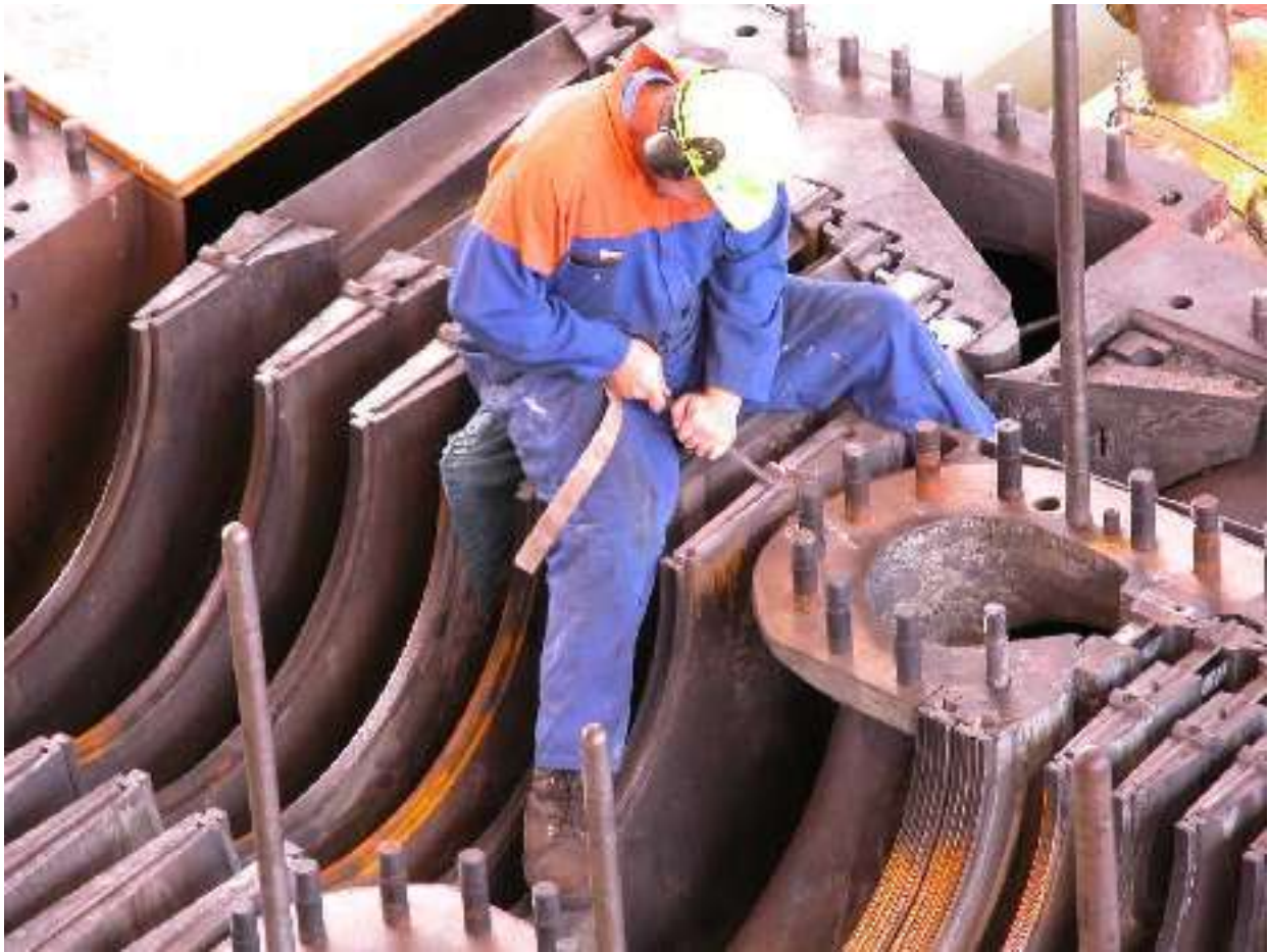
Scaring the old sealant away from the top of a diaphragm. A set of rotor blades fits in the gap between each.
