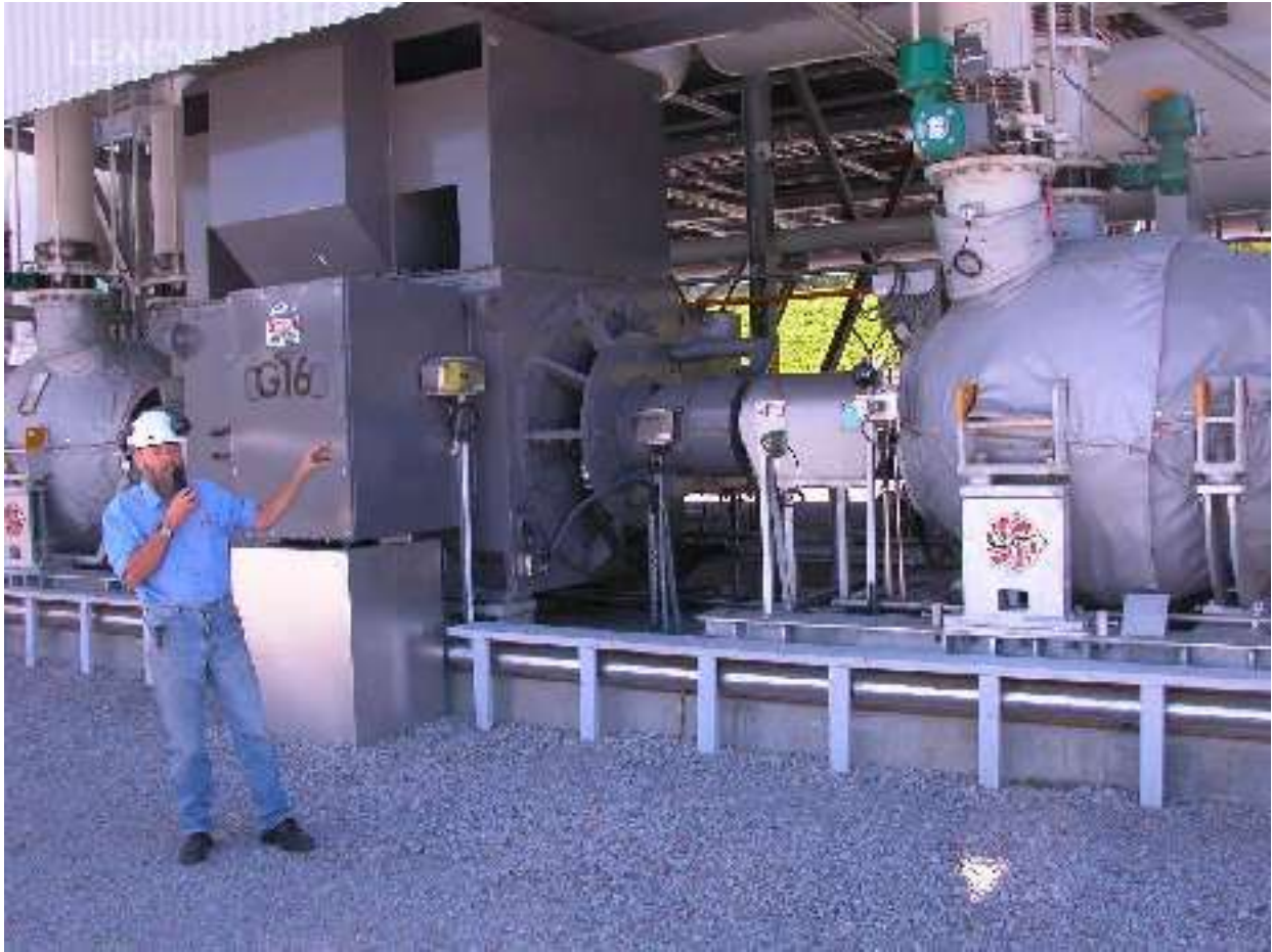
Chris explains how generator 16 is driven by the two, pentane gas driven, turbines
