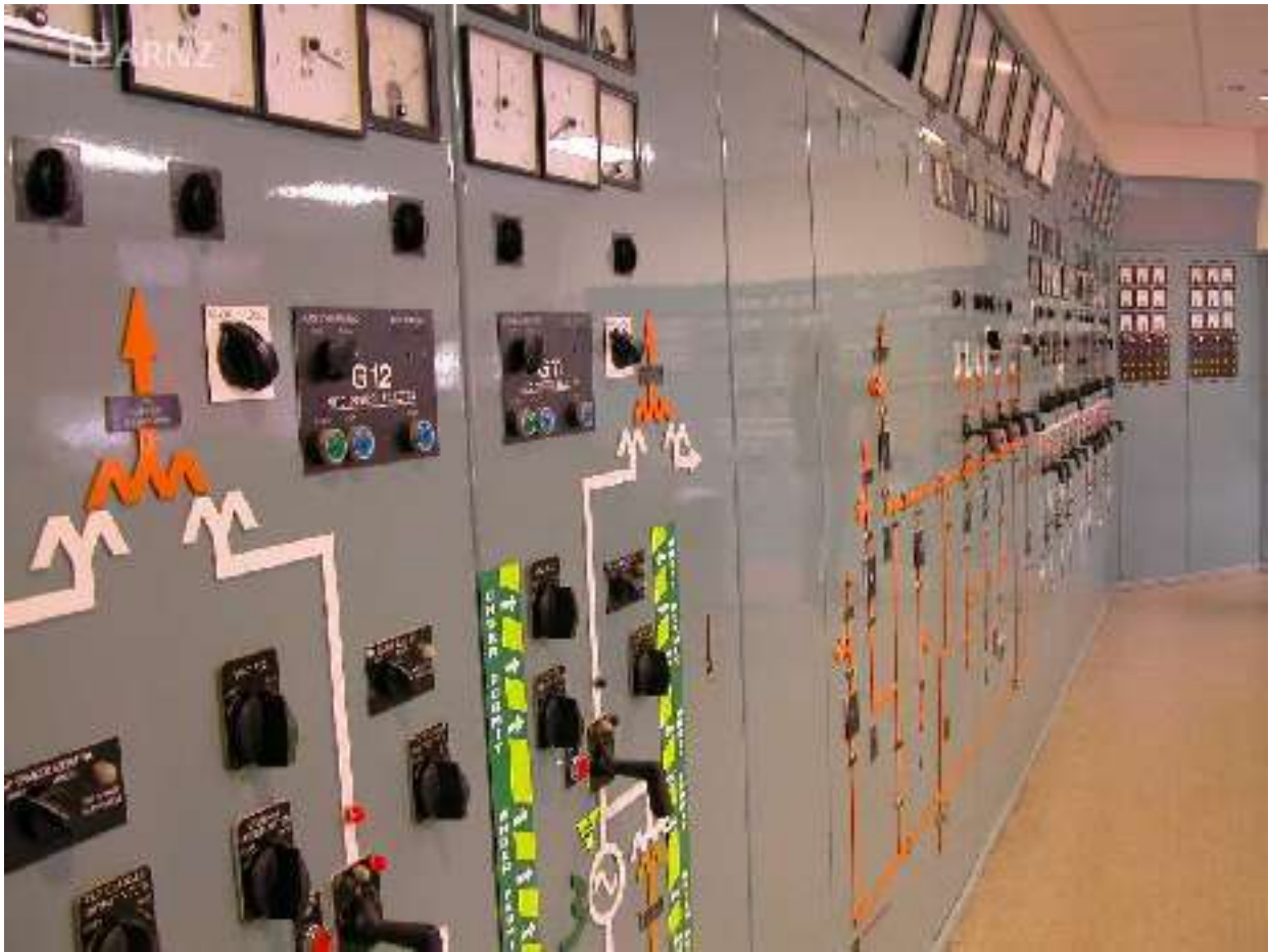
The original control board of Wairakei A station still works but is operated by remote computer networks now.
