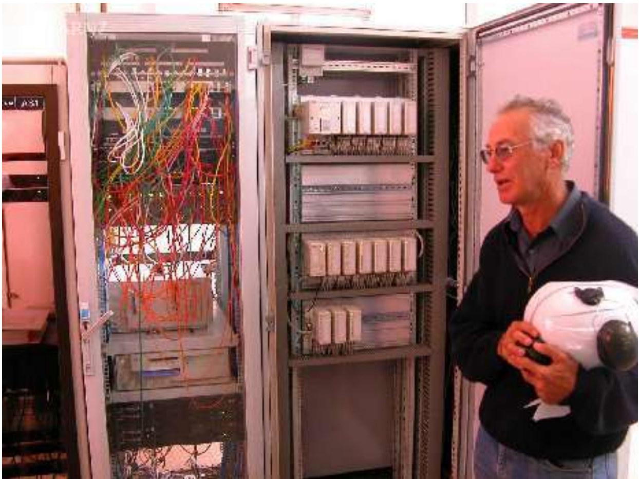
Murray Hill showing how Wairakei power station is controlled today by a computer network
